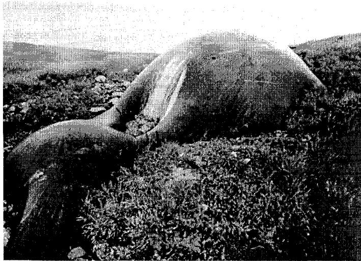
Figure 1.2 Localized inflation of a PVC membrane by gas pressure accumulated inside a landfill with restraint to inflation provided by topsoil coverage (after Koerner, 1994)
