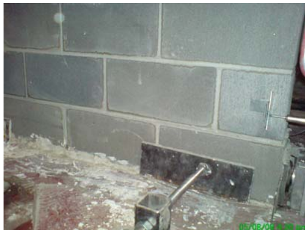
Figure 3.18: Rod and Steel Plates used on the Side of the Wall to Prevent Kicking Out
