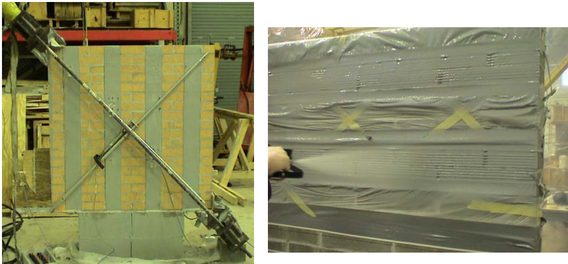
Figure 2.6: Test Setup (left) and Spraying Polyurea to one URM Wall (right) [Yu et al. 2007]
