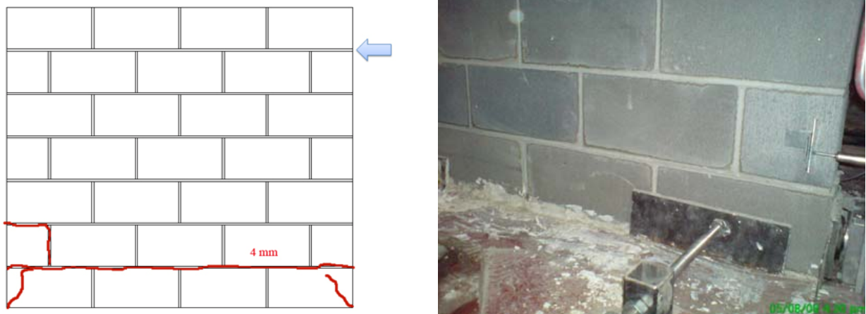
Figure 4.4: Cracks and Corresponding Displacement Cycle in Wall-S
