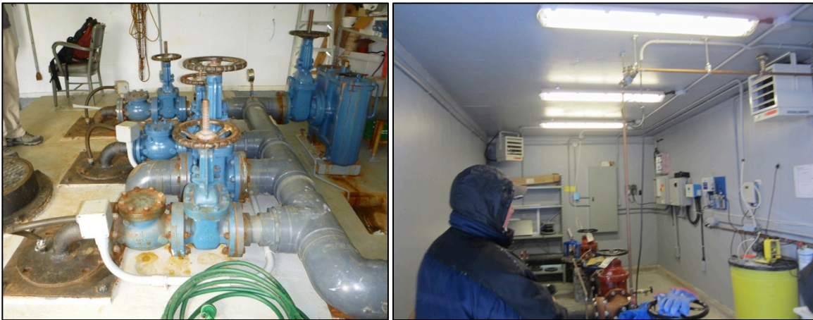
Figure 3.4. Examples of photos taken during field inspections. The photo on the right is of the interior of Rigolet’s main pump house. The photo on the left is of the interior of the building adjacent to the water storage tank that provides chlorination as water travels from the storage tank to users’ homes.
