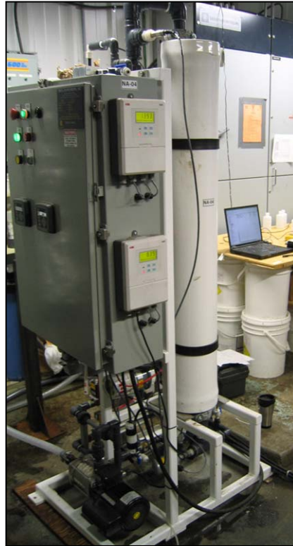
Figure 4-5 - Membrane filtration system used in Experiment I and III
